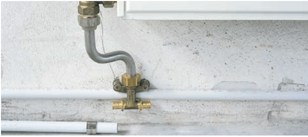
Installation T 16-V15-16
